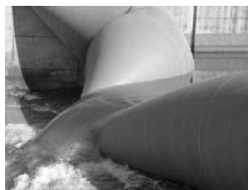
Figure 3: Buckling due to overflow
